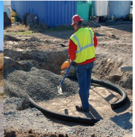
Step 3: Lay 100mm drain coil and first 150mm layer of 20mm road crush stone. Compact to 95%
