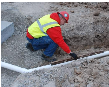
Step 7: Slope 90mm PCV storm water pipe away from foundation and run 25mm conduit from scale to controller. Back fill perimeter of scale, drains and conduit runs.
