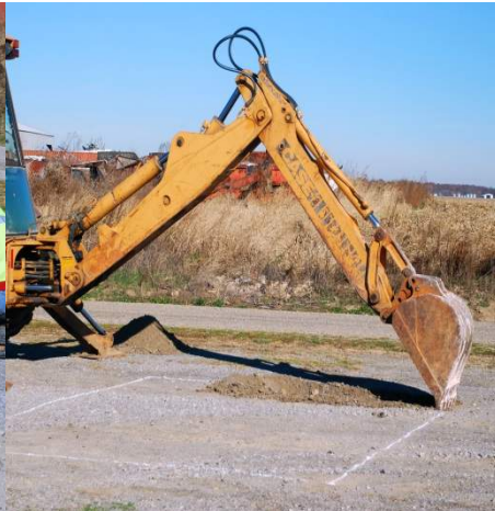
Step 2: Excavate and compact 4.2m X 3.2m x 0.6m deep. Dig a trench for home run cable and water drains.
