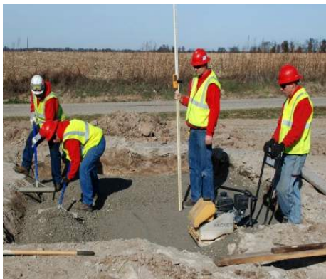
Step 4: Lay second layer of 20mm road crush stone, compact to 95%. Surface should be 295mm below grade or approach.
